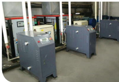
Energy recycling system
