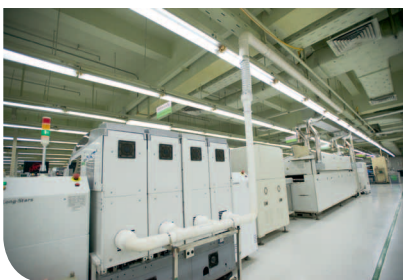
Extractors in infrared oven
